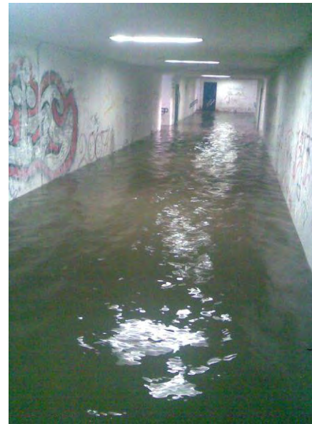
Figure 1. After intense rain water inundated the underground pedestrian passage under railway in Kostrzyn Wielkopolski in June 2010 (Kowalczak et al., 2010)
