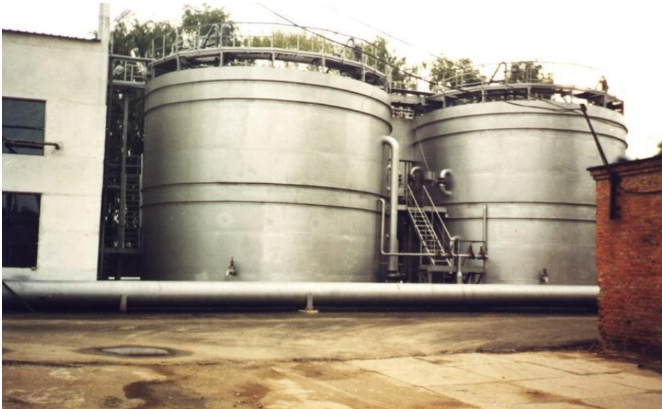
Fig. 2. Wastewater treatment plant of meat processing plant "Rhythm" in Chernihiv
