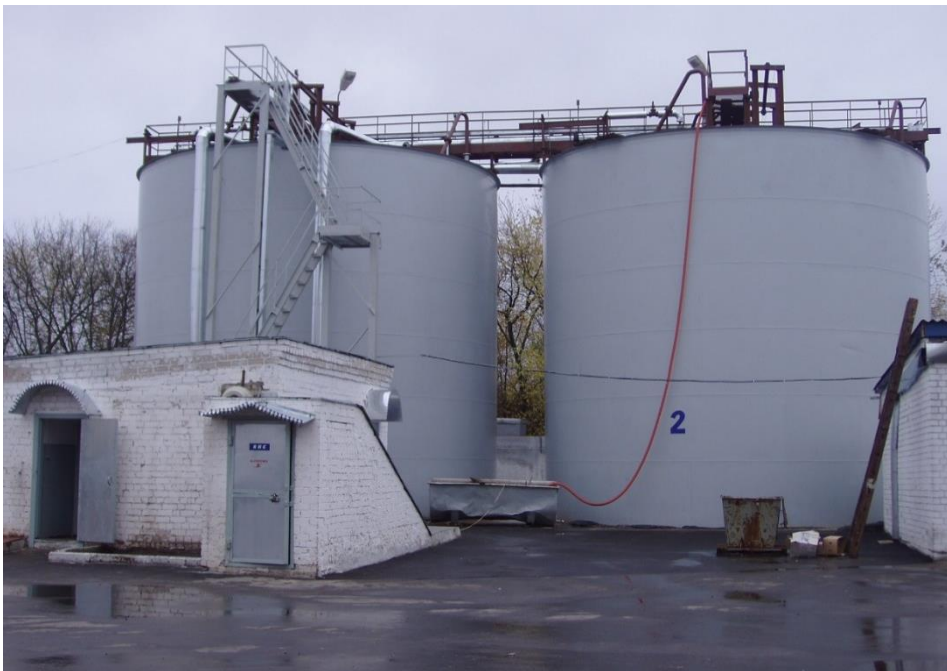
Fig. 3. Wastewater treatment plant of dairy processing plant in Shostka
