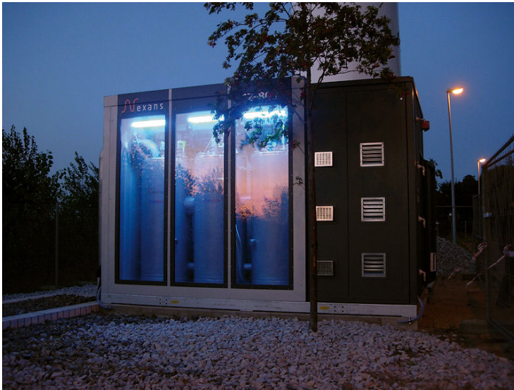
Fig. 2.17. Nexans HTS SFCL mounted in Boxberg power plant [11]
