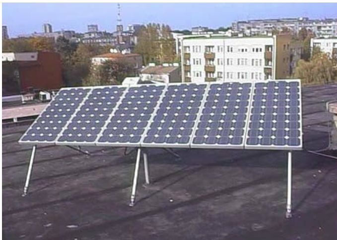
Solar battery of 6m 2 located on the roof of the building
