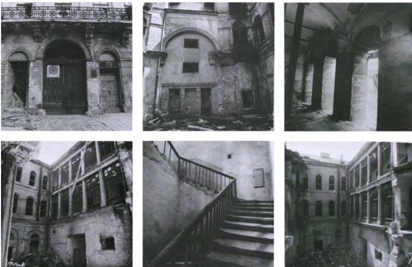
Fig. 5. The condition of the building at Mickiewicz Square 9 after the collapse of a part of the wall in 1997. Photo by I. Kostetskyi (Bevz, 2005)
