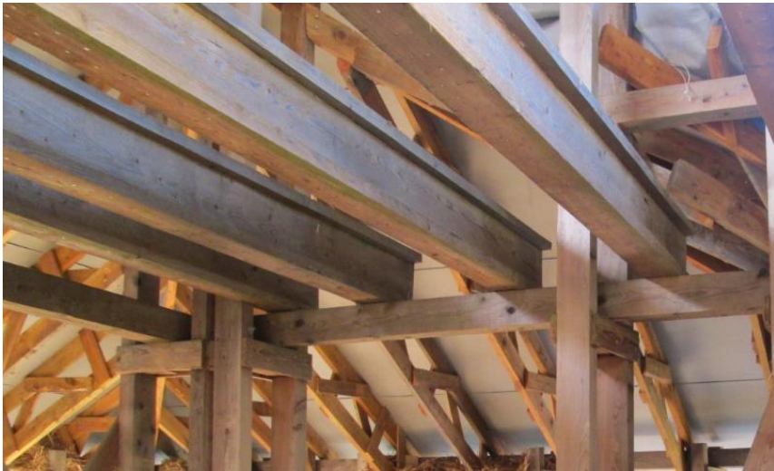
Figure 8.5. Composite double-T beams used as floor beams in residential building. Source: Author's archive
