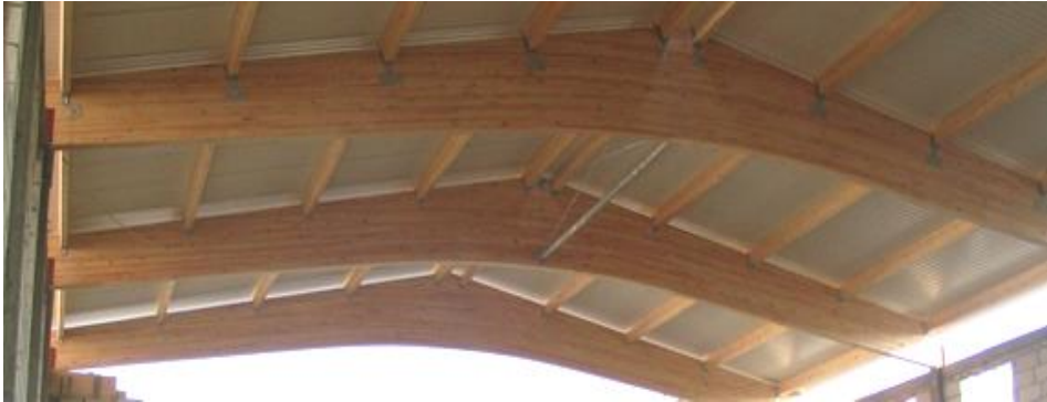
Figure 4.6. Pitched cambered beam of 18 m span in a school gym in Krasnystaw city, Poland. Source: Author's archive
