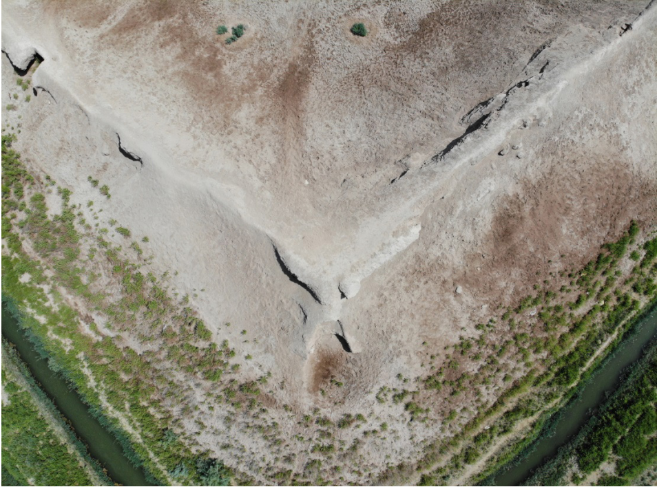
Fig. 4. Settlement of Kat-kala. View of the southwestern corner tower. Photo taken with a drone (B. Sadullaev, 2021)
