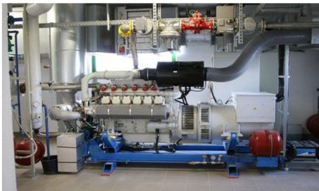
Fig. 3. Cogeneration power plant
