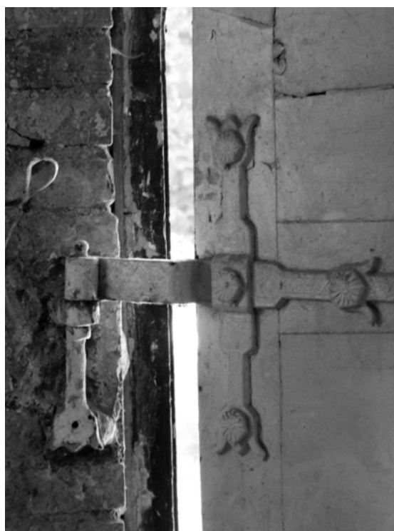
Fig. 8. Tatarów. "Straszny Dwór" guesthouse. Detail of the entrance door fitting in the Western façade. Photo J. Czubiński, 2012.
