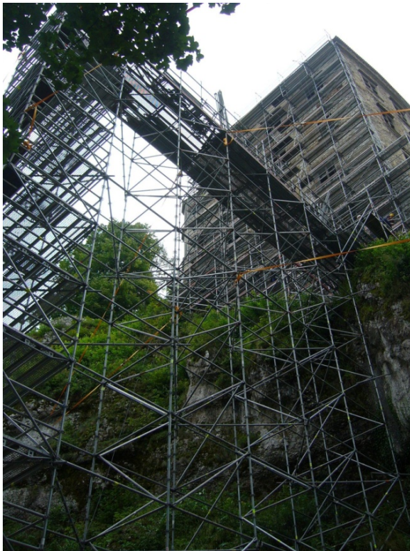
Fig. 2.9 The example of modular scaffold
