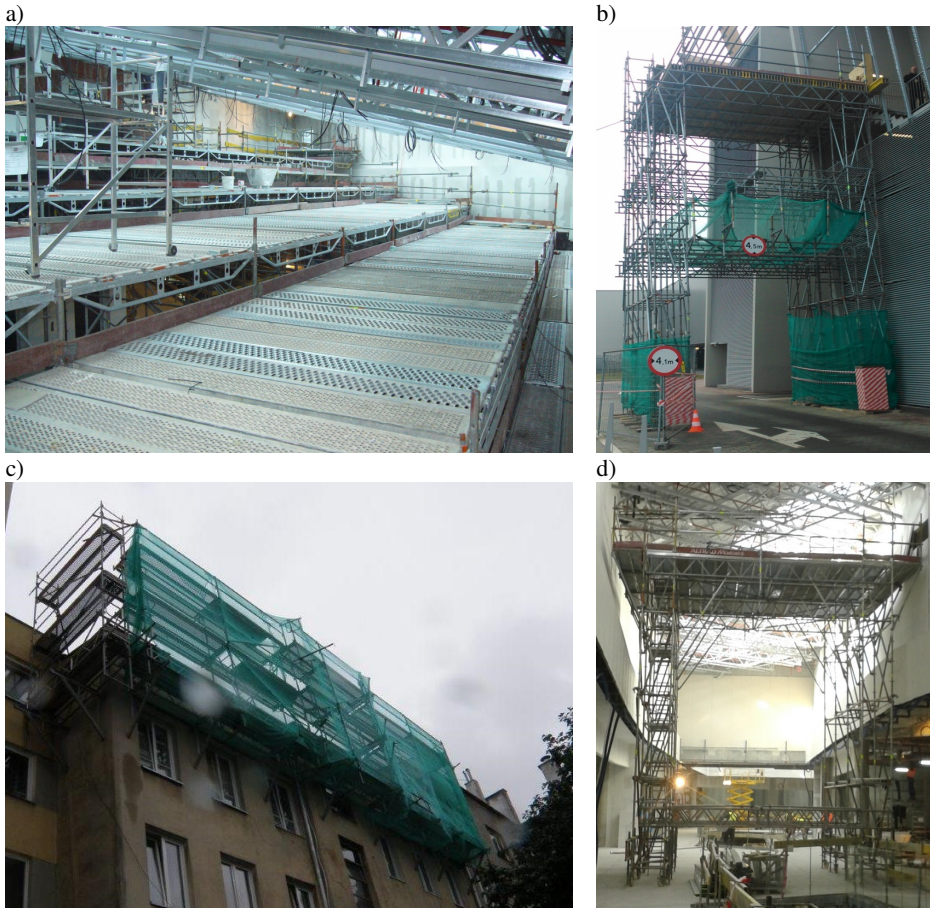
Fig. 3.1 The exemplary scaffolds: a) platform, b) platform for material, c) suspended scaffold, d) mobile platform
