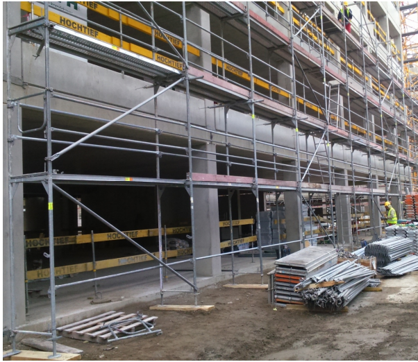
Fig. 2.8 The example of façade scaffold
