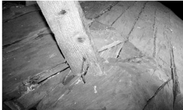
(Pic. 8) Renovation works carried out inappropriately in the rafter framing – threat to the construction of the property (photography depicting a wooden property inscribed on UNESCO's World Heritage List – yet, does not concern the churches in Lesser Poland Region), author: A. Sapeta
