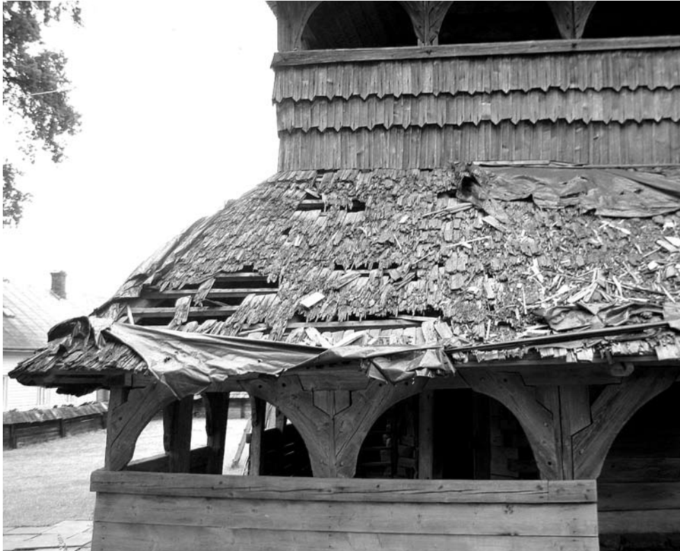
(Pic. 4) Complete destruction of the shingle roofing – threat to such attributes as material and construction (photography depicting a wooden property inscribed on UNESCO's World Heritage List – yet, does not concern the churches in Lesser Poland Region), author: A. Fortuna-Marek
