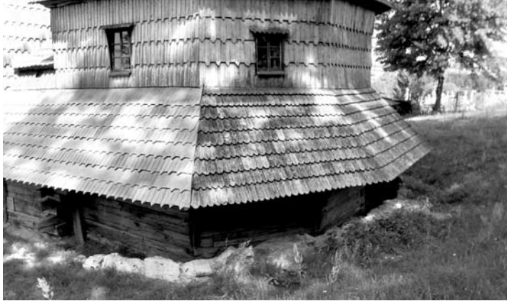
(Pic. 5) Inappropriate material applied to the roofing – plastic shingle (photography depicting a wooden property inscribed on UNESCO's World Heritage List – yet, does not concern the churches in Lesser Poland Region), author: A. Fortuna-Marek
