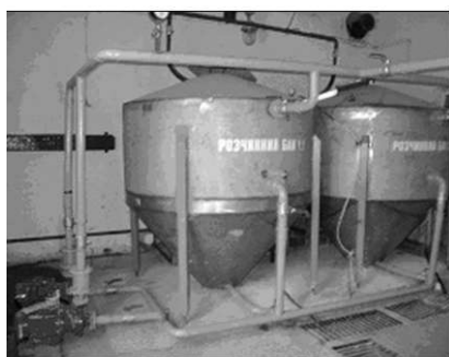
Recycling tanks of hydro mixers
