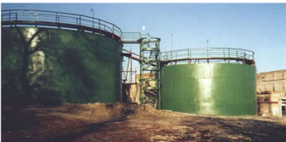
Fig. 5. Wastewater treatment plant of corn starch and caramel syrup production plant
