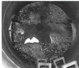
Fig. 6e. Condition: bad
