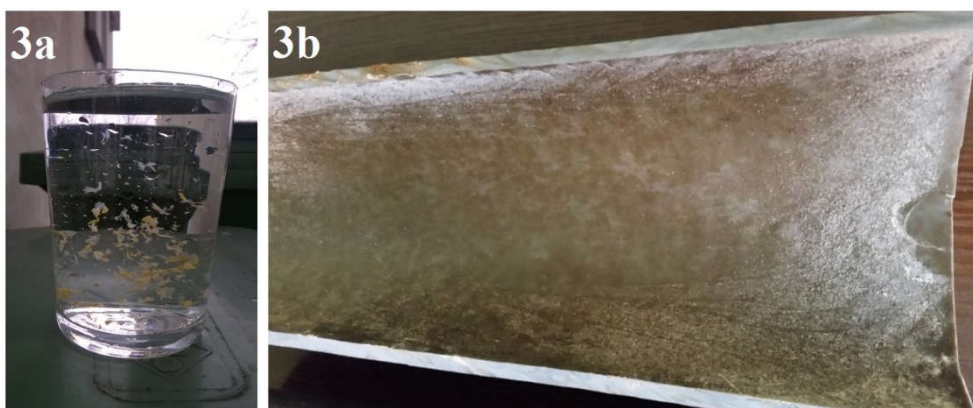
Fig. 3a) Water sample extracted from water supply network measuring point 2 Fig. 3b) Internal surface of PVC-U pipe (DN160, year of building: 1985) extracted from an existing water supply network
