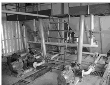
Clarifiers - recyclers of working solution
