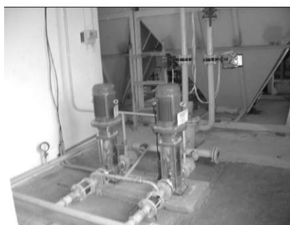
Dosing pumps with pH controllers of working solution
